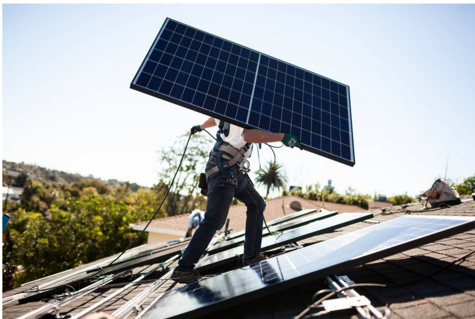
A worker carries a solar panel into place at a customer's home in Carlsbad, Calif., Oct. 18, 2018.
